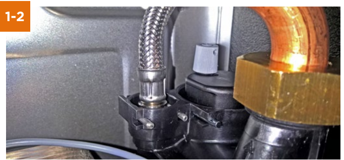
Flue system is all connected, auto air vent in the boiler is open.
