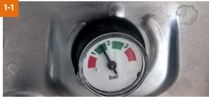
All boiler isolation valves are open, system pressure is between 1.50 – 2 bar.
